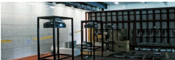
Three PT-D5700L projectors are installed behind the screen.
