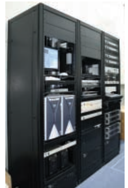
Two hard disk servers are mounted on an equipment rack.
